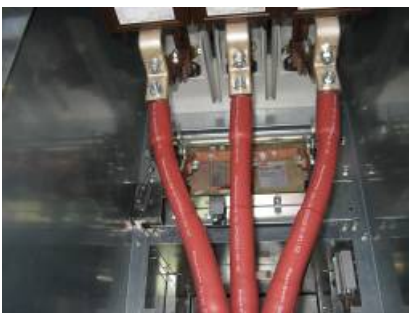
Internal view of the cable connection compartment.
